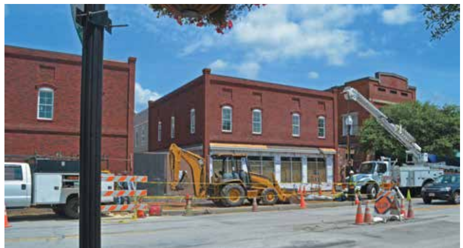
The Mantissa is a boutique hotel under construction in Hartsville. (Photo: City of Hartsville)
